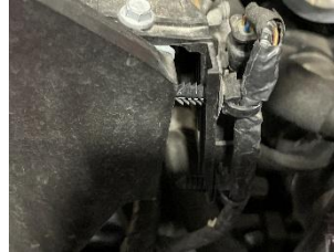
Figure 12: Fir Tree fasteners retaining wiring harness to passenger side battery tray.
