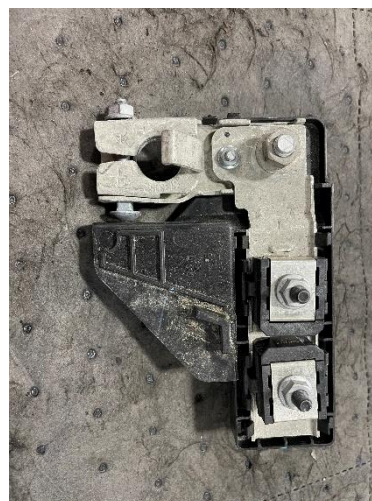
Figure 10: Positive terminal cluster removed.
