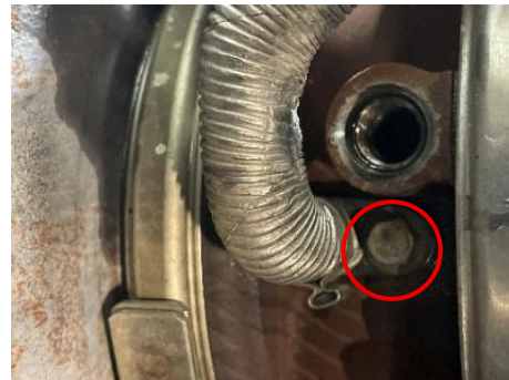
Figure 23: Turbine shaft speed sensor installed in turbocharger. 8MM bolt retaining the sensor circled.
